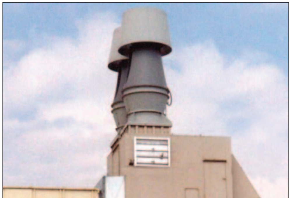
A typical Tri-Stack system with accessory heat recovery unit.
