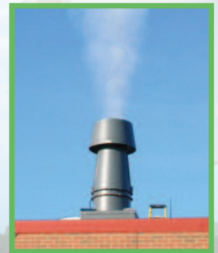
High dilution makes the Tri-Stack® ideal for exhausting diesel generator fumes.
